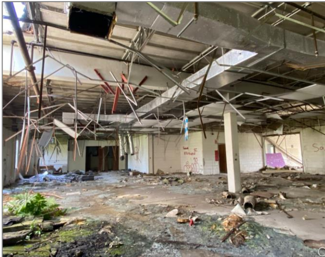
View of the inside of a heavily damaged building within the San Juan Metro area
