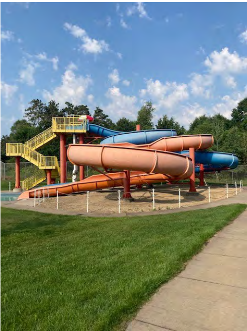
Splash Cove Water Slide needs refurbishment. Scheduled for 2024.
