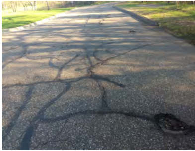
Existing road conditions proposed for reconstruction at Bunker Hills Regional Park
