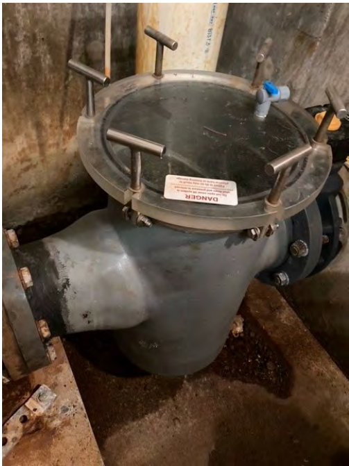
This is an on-going project that proposes to replace a certain number of strainers each year going forward. This also includes plumbing improvements and sand/silt well filter installation.
