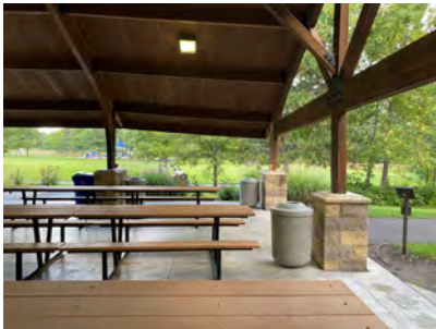
Pavilion One and Three proposed for replacement due to structural issues.
