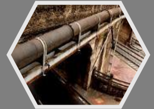
OVER 20,000 MILES OF PIPES Water & wastewater
