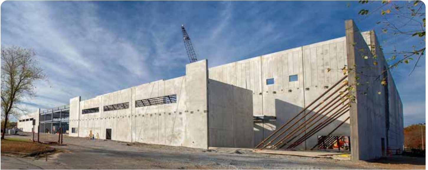
Pictured above is construction on the new Henrico Sports and Entertainment Center at Virginia Center Commons. The facility will be about 185,000 square feet, featuring 12 basketball courts or 24 volleyball courts, an arena with stadium seating, and 3,500 fixed seats. It can expand to about 4,500 seats for graduations, concerts, or special events. The design allows for different types of events to go on at the same time. The facility will provide more opportunities for residents and a boost for sports tourism. Completion is anticipated in 2023.
