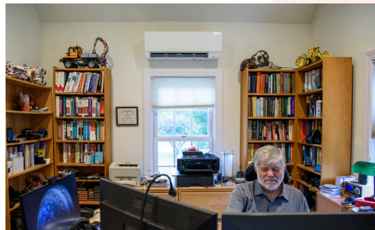
Bill added a ductless heat pump to his home office to increase year-round comfort and efficiency.
