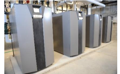
Modern Condensing Boiler With Higher turndown
