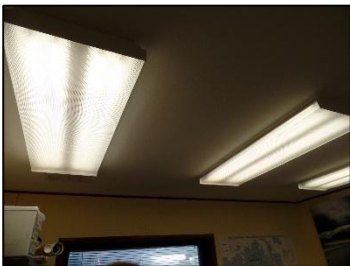
Existing Solid Waste T8 Lighting
