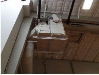
Gymnasium Air Handler
