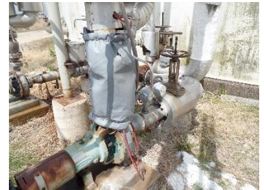
Pump Station at Venture Park Holding tank
