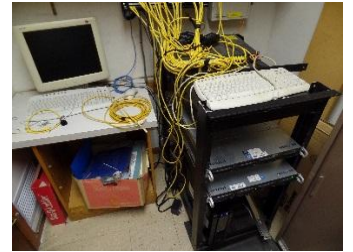
Server Closet at Vehicle Maintenance Garage Office
