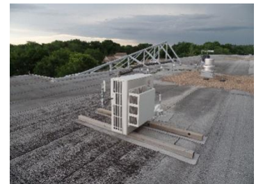
Substantial De-Mineralization on Community Health Building Roof
