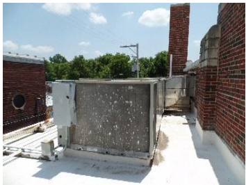
Rooftop Hail Damage
