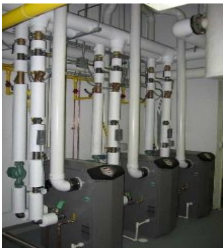
Central Hot Water Plant
