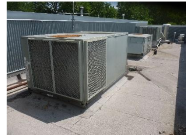
Older RTU at FS#2
