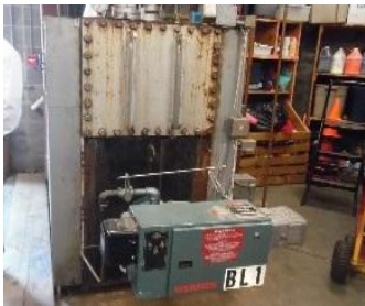
Aging AJAX Boiler
