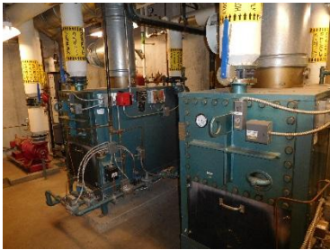
Existing Atmospheric Boilers
