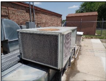
Solid Waste HVAC Unit
