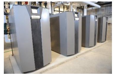
Condensing Boiler Plant
