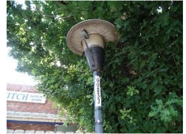
Aged and Distressed Pole To Be Replaced
