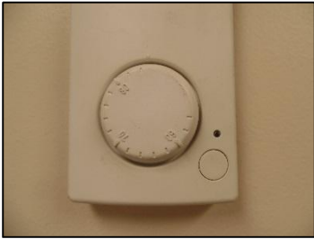
Existing DDC thermostat
