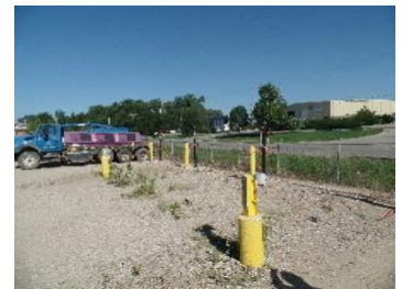
Block Heater Receptacles on Bollards
