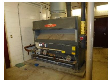
Pool Water Heater
