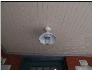
Exterior Depot Lighting
