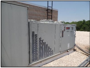
Packaged rooftop unit
