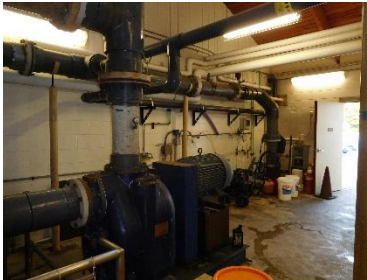
Pool Recirculation Pump
