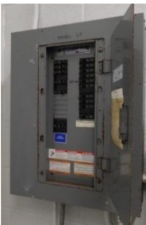
Panelboard with Corrosion
