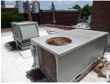
Existing Packaged Unit (1993)
