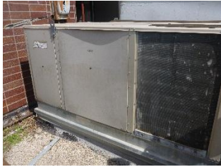
Older RTU at FS#3
