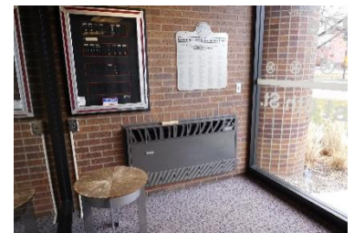
Electric Cabinet Heater at Main Entry
