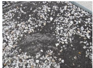
Roof deterioration at FS#3
