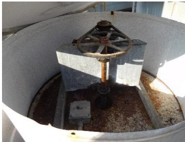
Decommissioned Exhaust Fan
