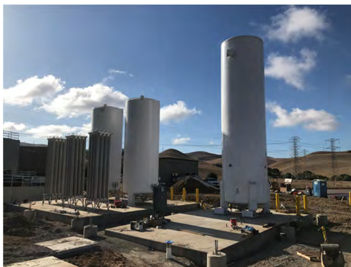
New liquid oxygen and carbon dioxide tanks at the DVWTP Ozone facility.
