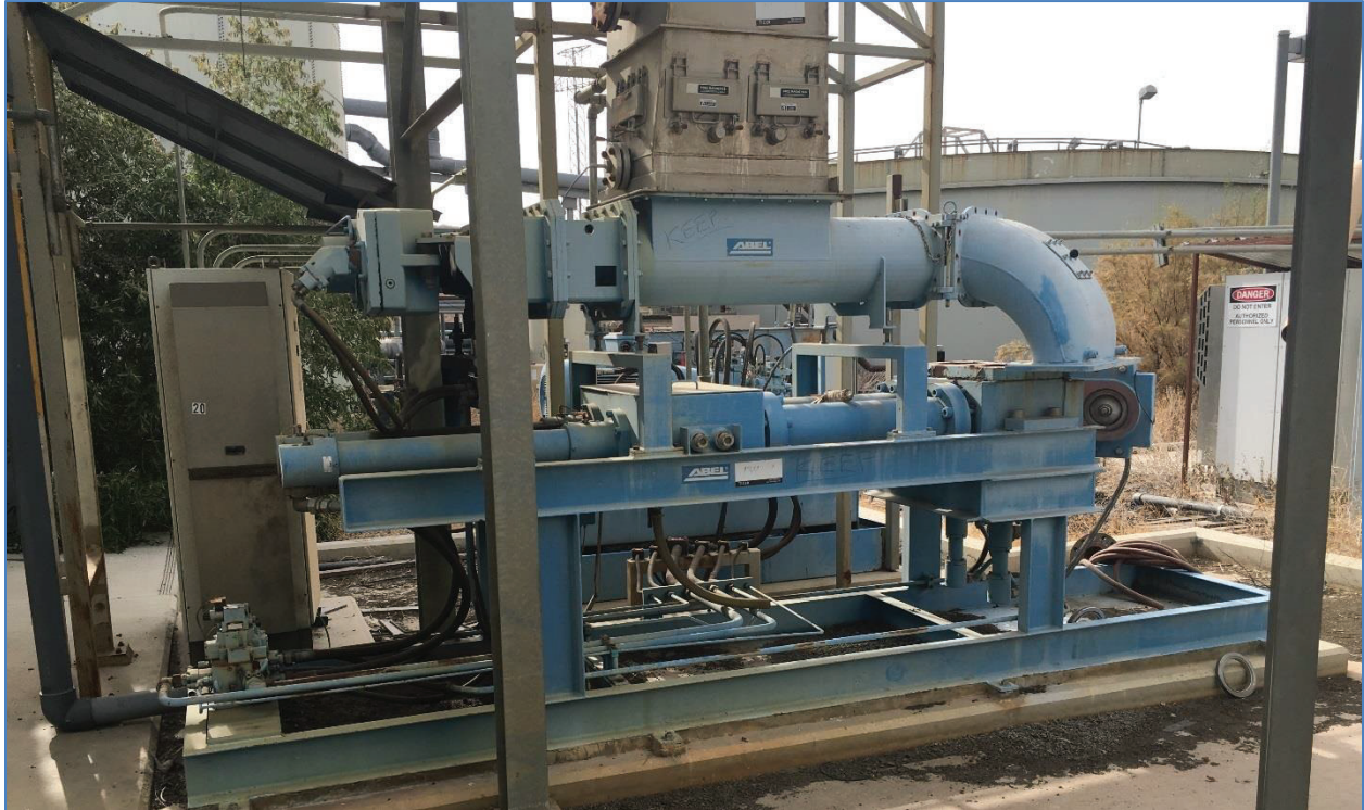
Figure 2-6 Existing High-Pressure Feed Pump
