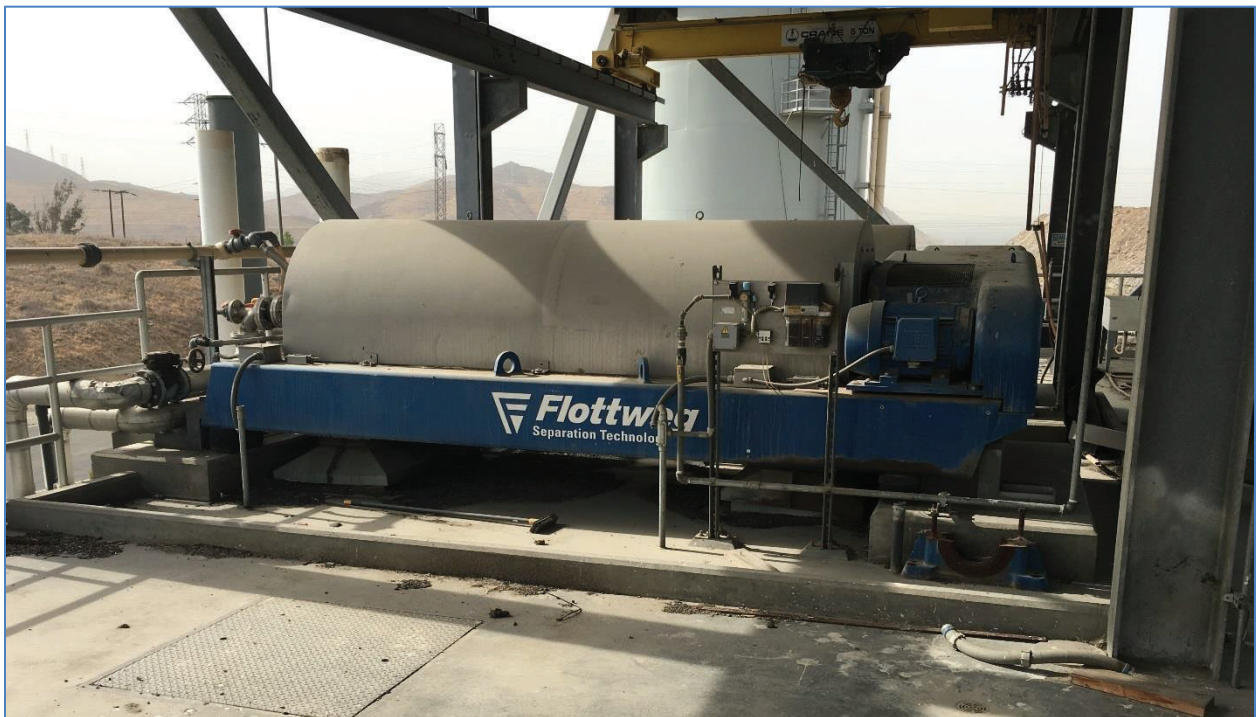
Figure 2-7 One of Two Existing Centrifuges
