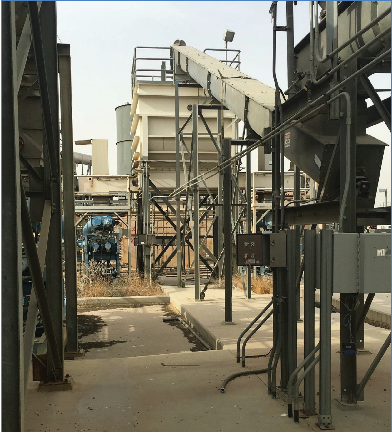
Figure 2-5 Existing Transfer Screw Conveyors and Cake Blending Bin
