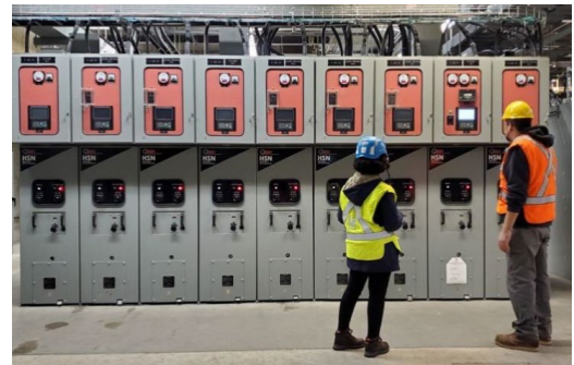
Inverter cabinets for railcar braking energy recovery (Pictured: Van Dorn St traction power substation)
