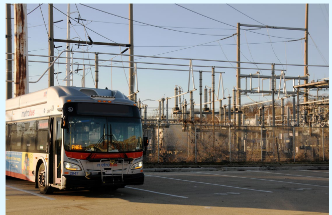
Metrobus in front of electric utility substation (Pictured: Bus parked at Four Mile Run Bus Garage)
