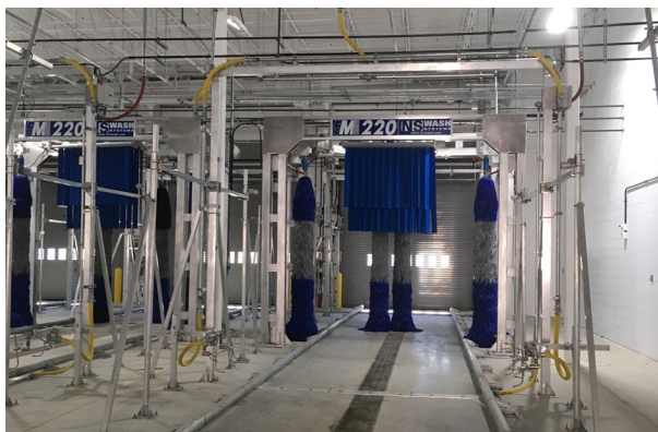
New bus wash bay at Andrews Federal Bus Garage reduces energy and water consumption.
