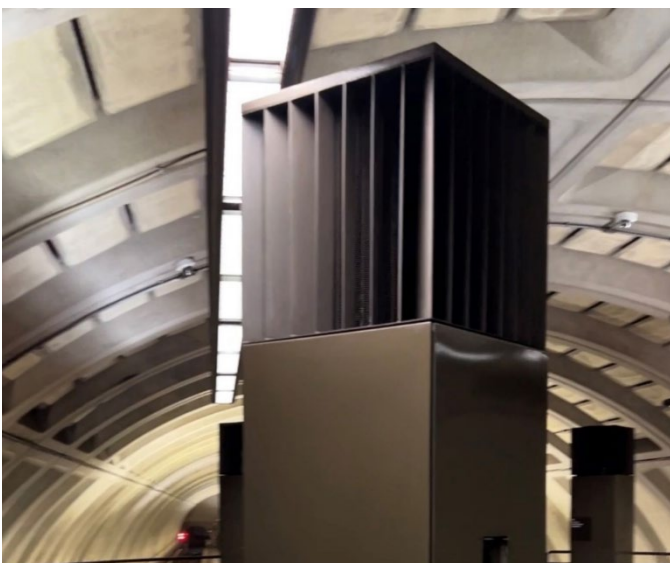
Underground Metrorail station cooling system
