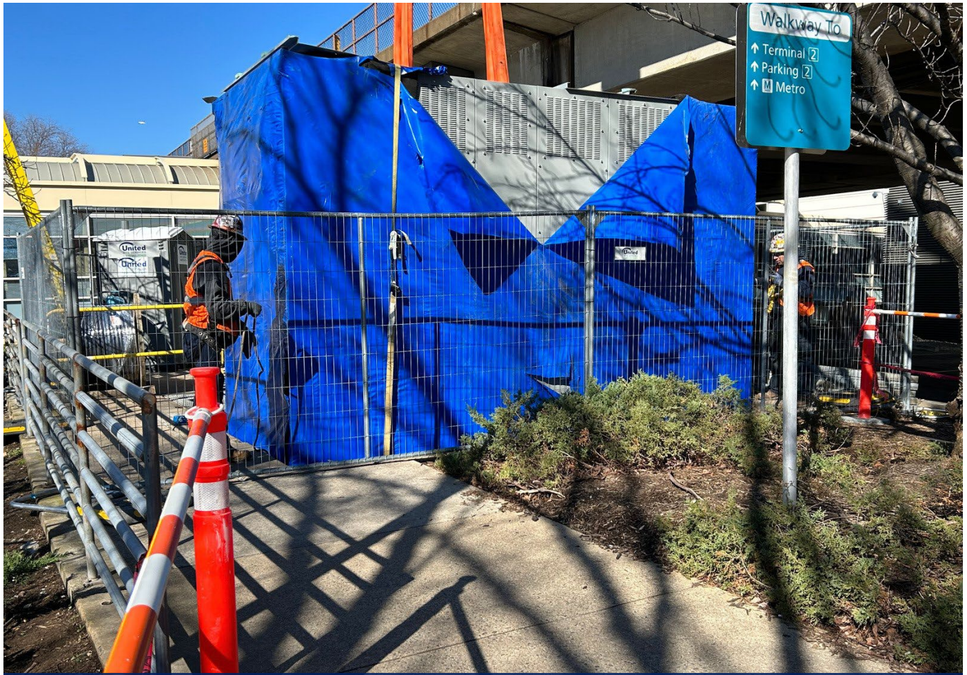
Metrorail traction power upgrade on Blue and Yellow line in preparation for Potomac Yard station
