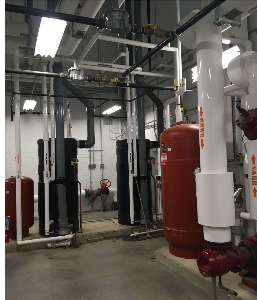
Energy and water efficient boiler at Andrews Bus Garage
