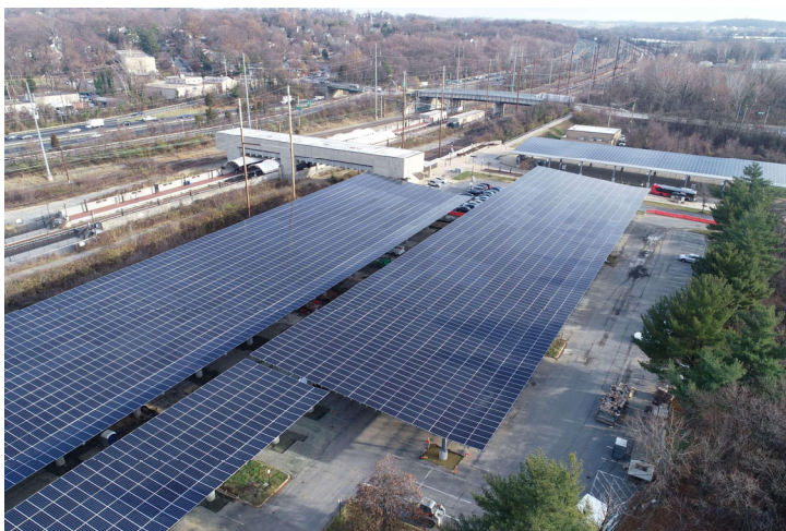
Pictured: Solar carports at Cheverly Metrorail Station
