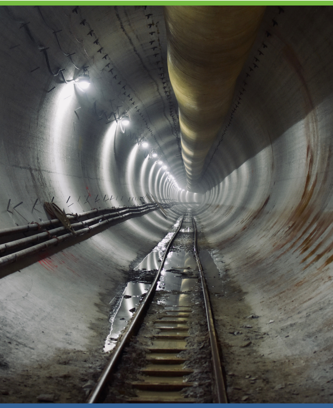
MSD's 4-mile Waterway Protection Tunnel will protect the community and our waterways from combined sewer overflows.
