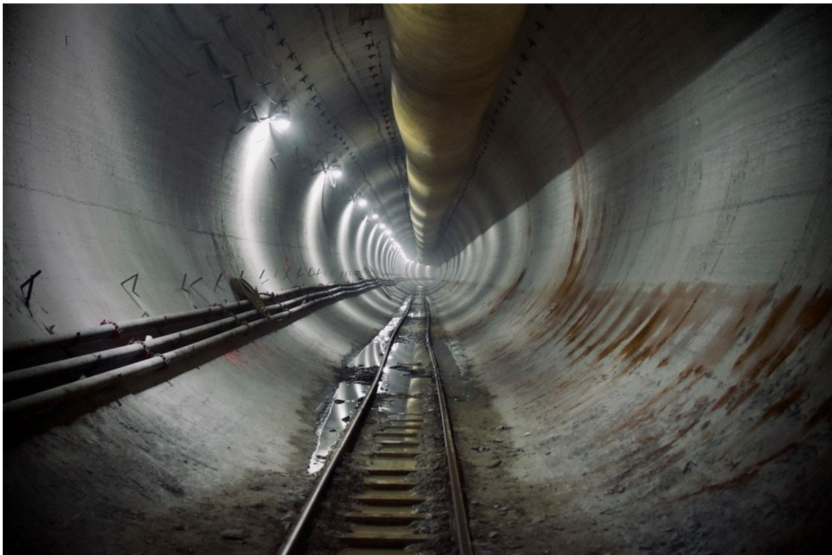
MSD's Waterway Protection Tunnel.
