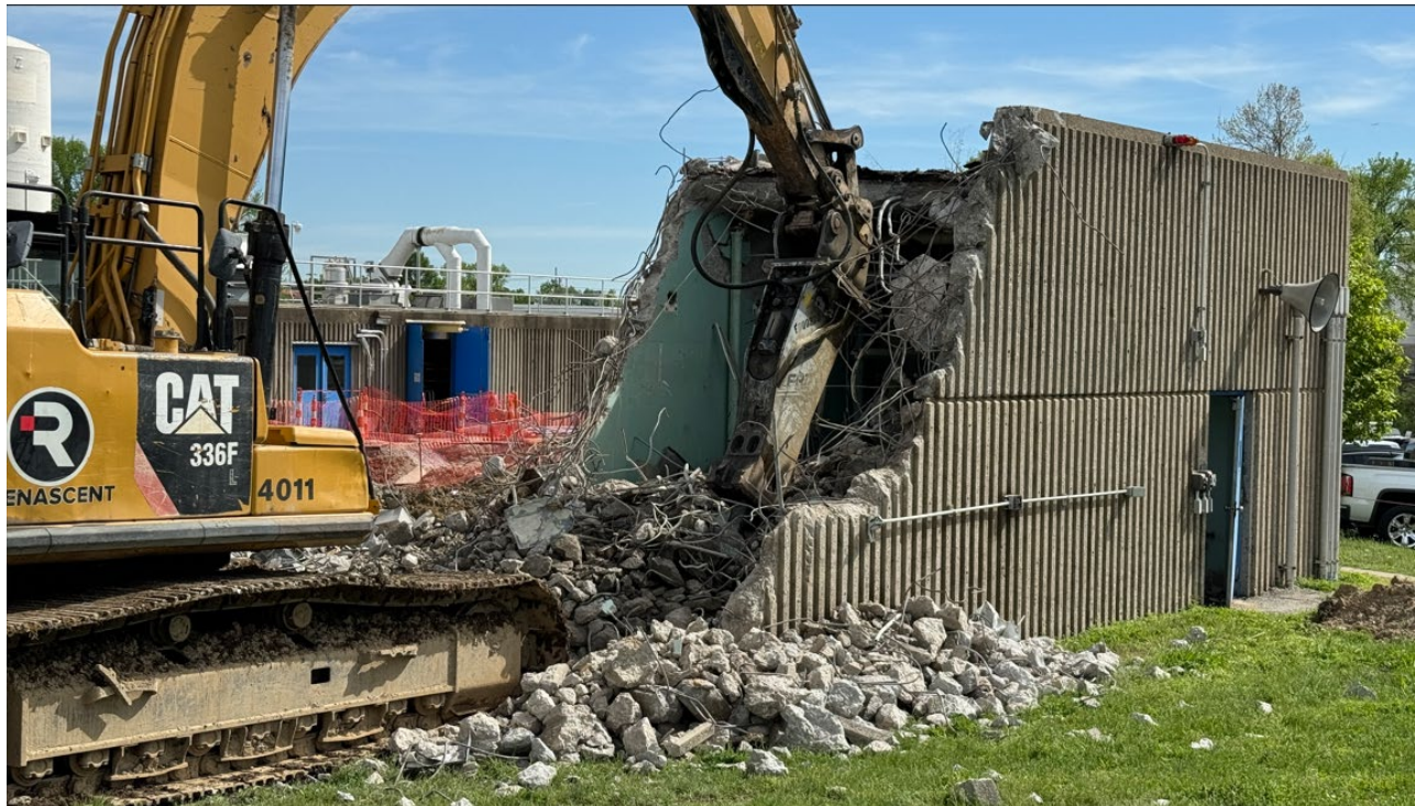
Demolition is underway at MFWQTC in preparation for the new Biosolids facility.
