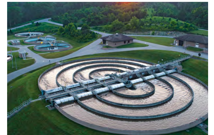
Floyds Fork Water Quality Treatment Center
